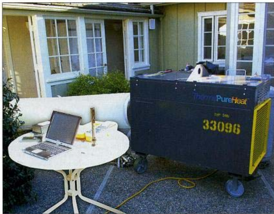
Insurers and property owners are finding that heat offers an effective alternative or adjunct to costly traditional demolition-based mold remediation and flood restoration. Heat treatment can raise temperatures in targeted areas or entire structures to levels lethal to biological pests.
